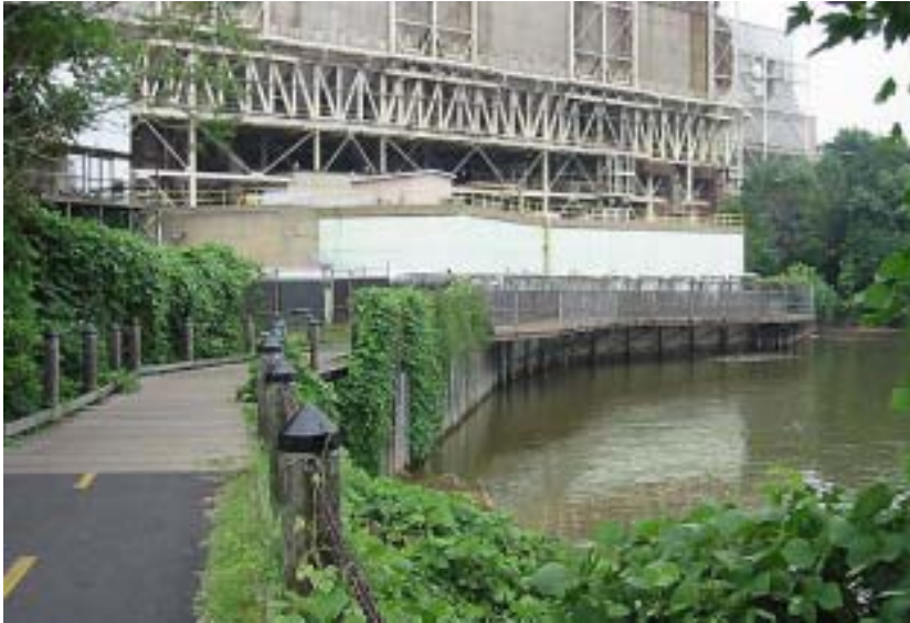
Example of a trail supported along a retaining wall on Mt. Vernon Trail at the Alexandria Power Plant
